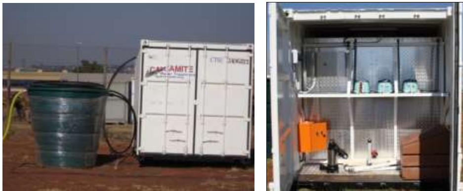
Fig 19: Containerised waste water treatment plant
