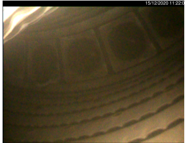
Picture 19: combustor outer liner
