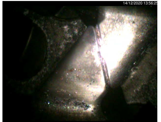
Picture 2: mid span damper
