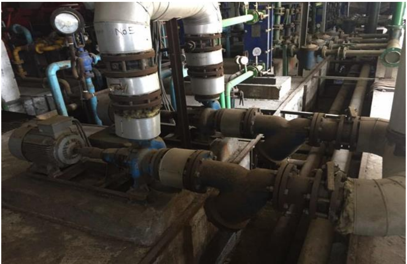
Technical Details & Photographs Of 2 Nos. 1000 kW Waukesha make Gas Generator Sets
