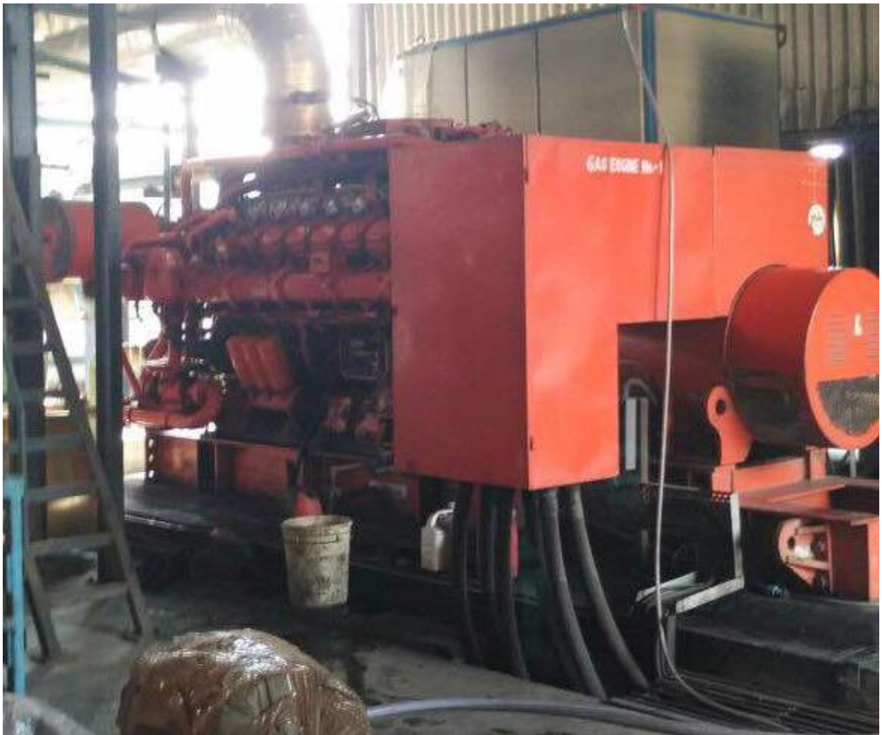
Technical Details & Photographs Of 2 Nos. 1000 kW Waukesha make Gas Generator Sets
